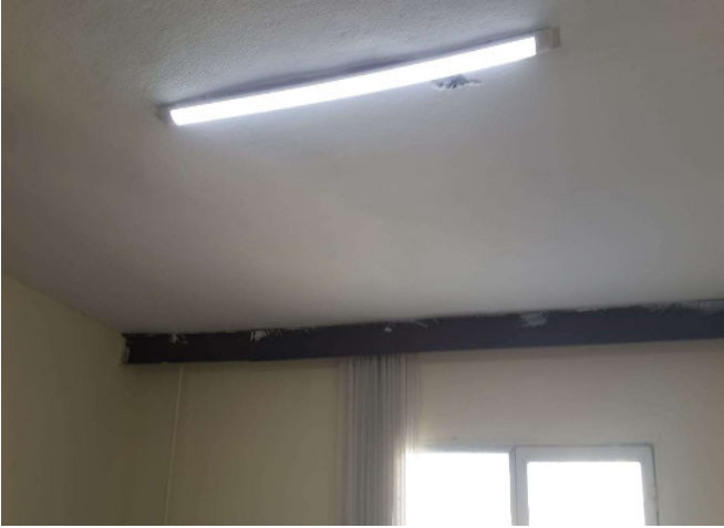
LED floresan aydınlatma (beton tavan)
